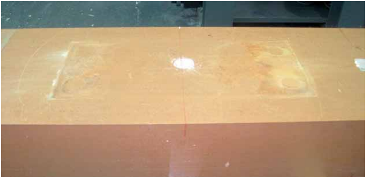
Only slight plastic deformations were ascertained under the rail supports
